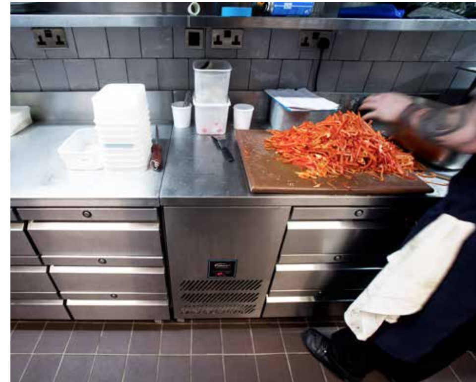
Blast Chillers and Refrigerated Counters Beaumont Hotel
