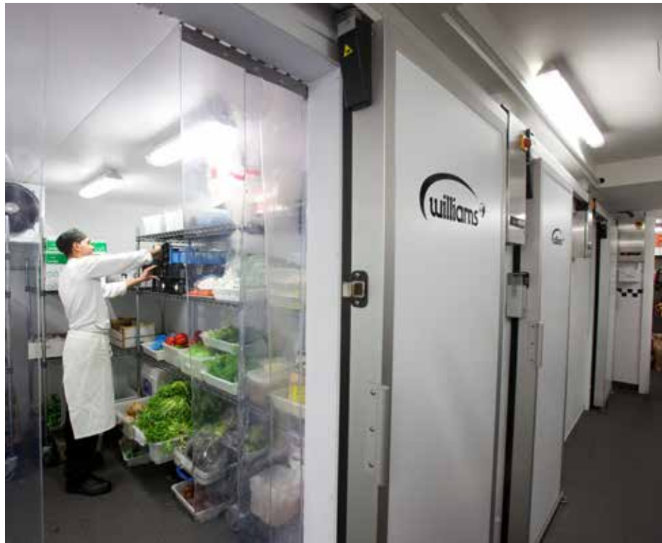
Modular Refrigeration and Coldrooms Le Cordon Bleu
