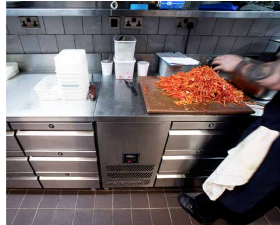
Blast Chillers and Refrigerated Counters Beaumont Hotel
