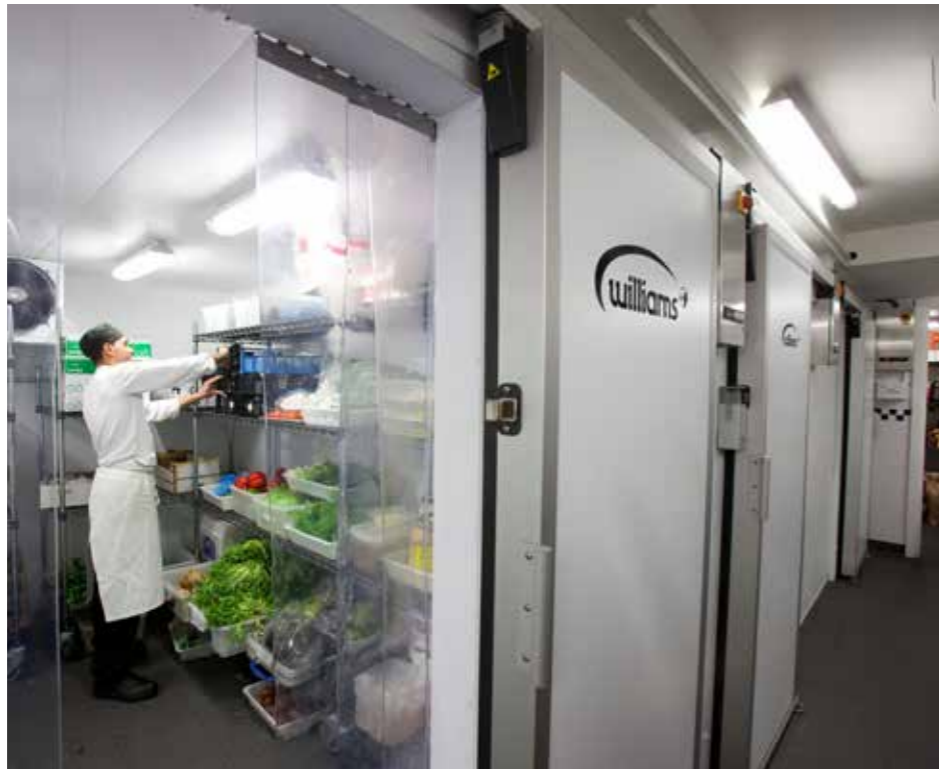
Modular Refrigeration and Coldrooms Le Cordon Bleu
