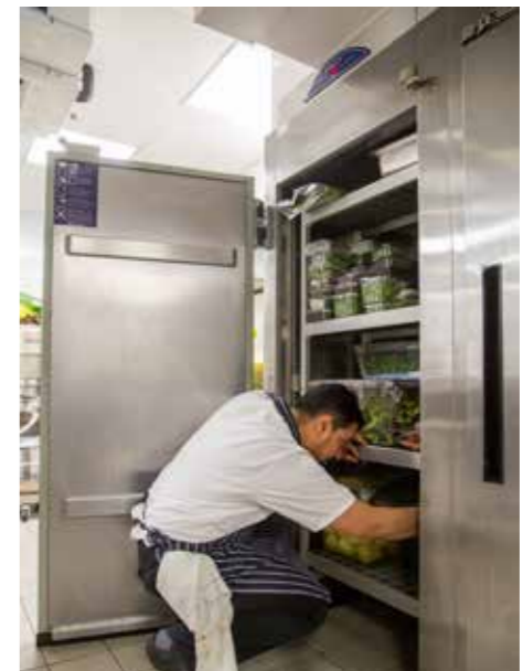
Counters, Coldrooms and Modular Refrigeration Sea Containers
